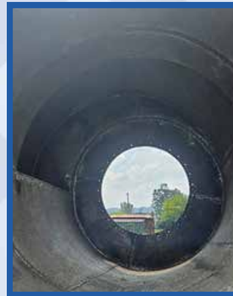
Cyclone fabricated with mild steel and then rubber lined with liners fitted afterwards.
